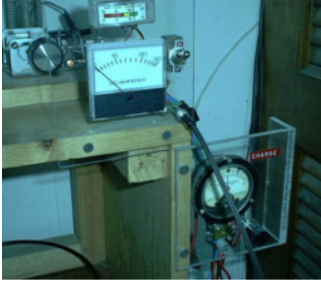
Battery charge monitor
