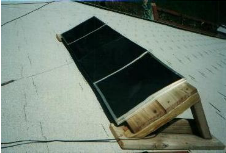
Solar panel on the roof
